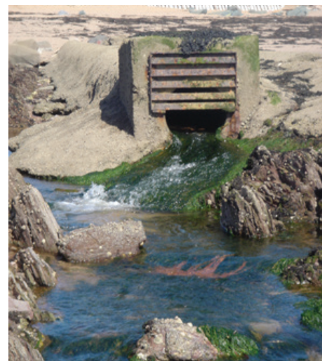
Sewage outfall - the Thurstlestone stormwater overflow (photo: Tom Hutchinson)
