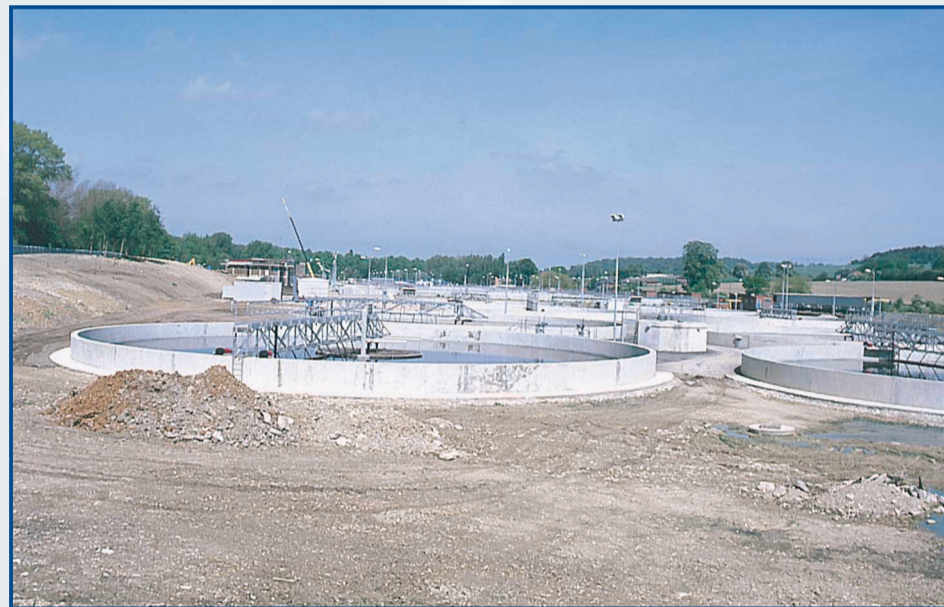
A sewage treatment works
